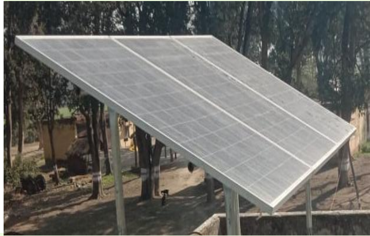
15 Solar Power Unit & 12 Solar Water Pump
